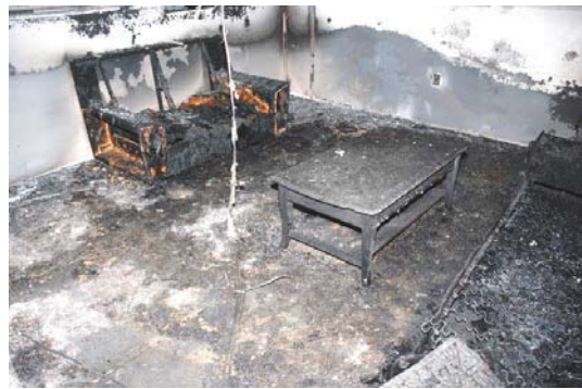
Figure 23: Post Fire Damage
