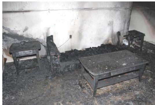
Figure 23: Post Fire Damage
